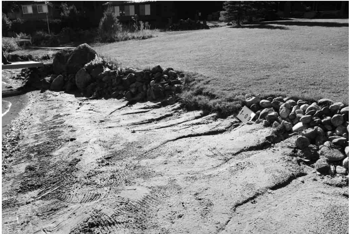
This erosion on McGrath Pond-Salmon Lake is from water flowing across a sloping lawn with no other vegetation to slow the runoff. Grass does not absorb runoff well and is less effective at holding dirt in place.
